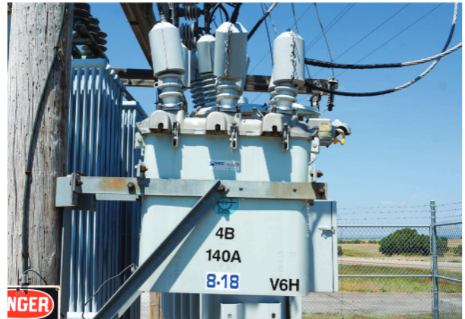
Currently, Prairie Land uses reclosers without electronic controls.
