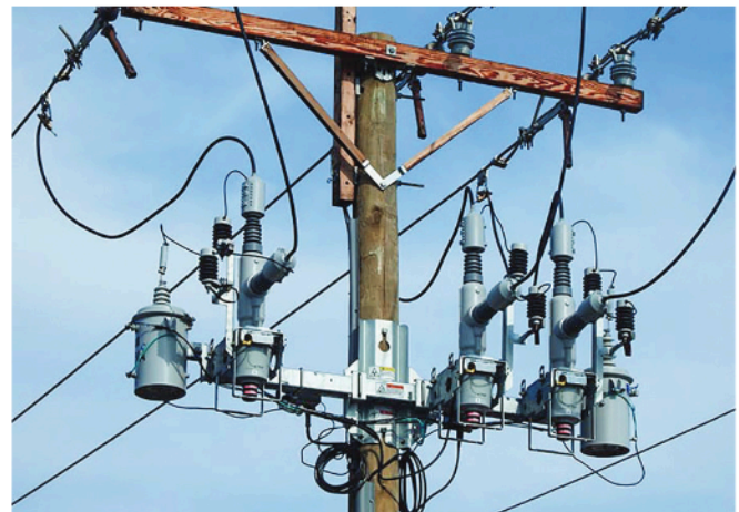
To improve our system reliability, Prairie Land will be installing automatic circuit reclosers with electronic controls.
